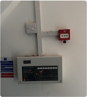
3.3.6 - Fire Alarm Panel
